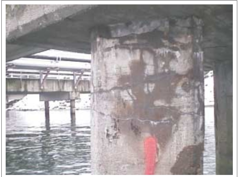
Example of a cracked concrete pile in the oilharbour at Södertälje.
